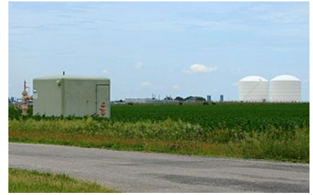
Peoples Gas Manlove Field natural gas storage area in Newcomb Township, Champaign County, Illinois. In the foreground (left) is one of the numerous wells for the underground storage area, with an LNG plant, and above ground storage tanks are in the background (right).
