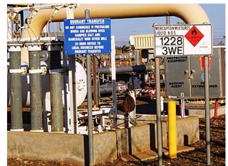
A pipeline odorant injection station
